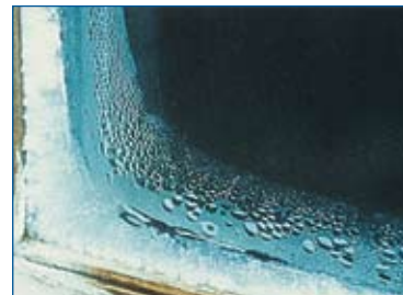
Window condensation can fuel mold growth.
